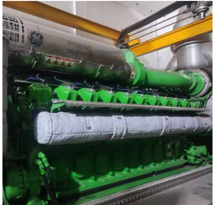
INNIO Jenbacher JMS 620 Type J gas engine at Suraj Cotton Mills Ltd, Raiwind, Punjab.
